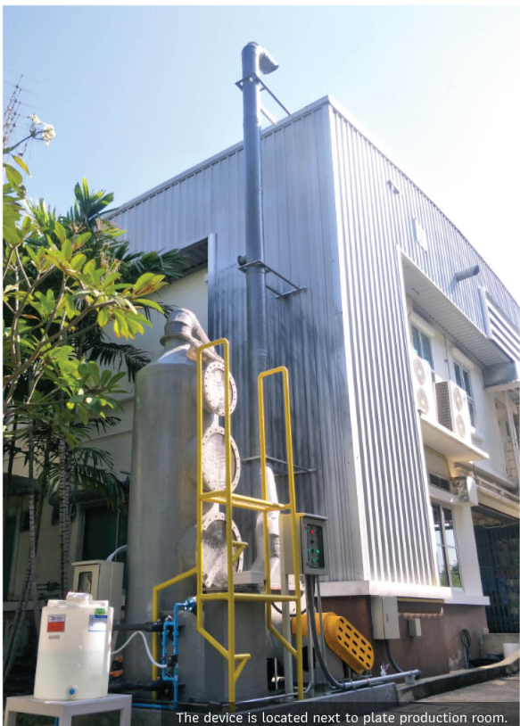
The device is located next to plate production room.
