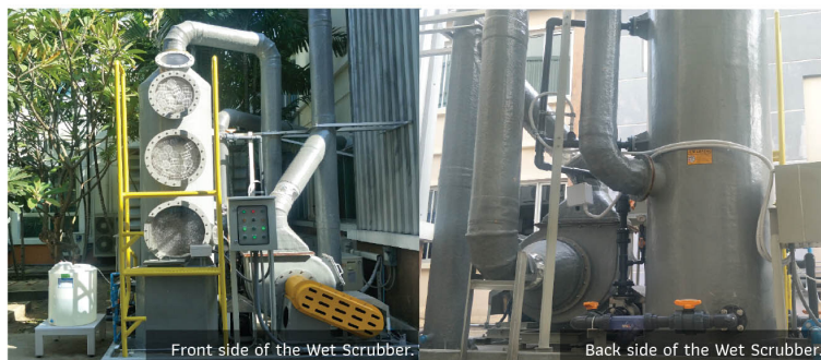
Front side of the Wet Scrubber.
